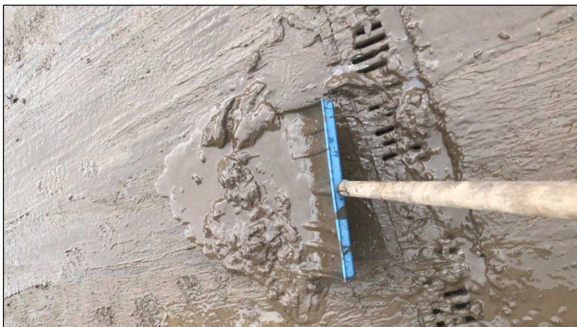
Figure 12: Photo shows deposits of mud blocking the surface water drainage infrastructure at Park Lane following the flooding during Storm Dennis (image provided by resident)
